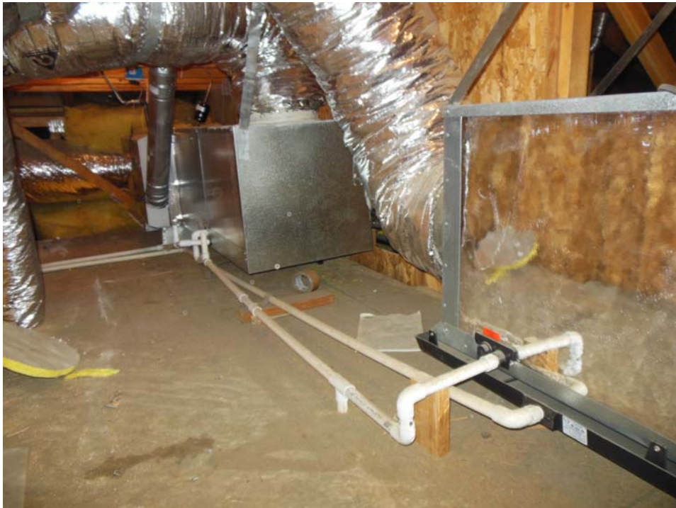
View of good quality and neatly installed Carrier brand HVAC units in attic space. Both units came on in heat mode and were also cooling properly in cooling mode. The installations are neat and tidy.
