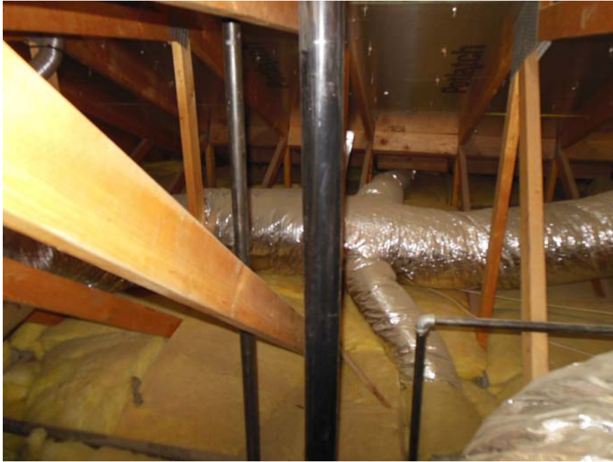
Another attic view. Note neatly and good quality heating and cooling duct systems installation.
